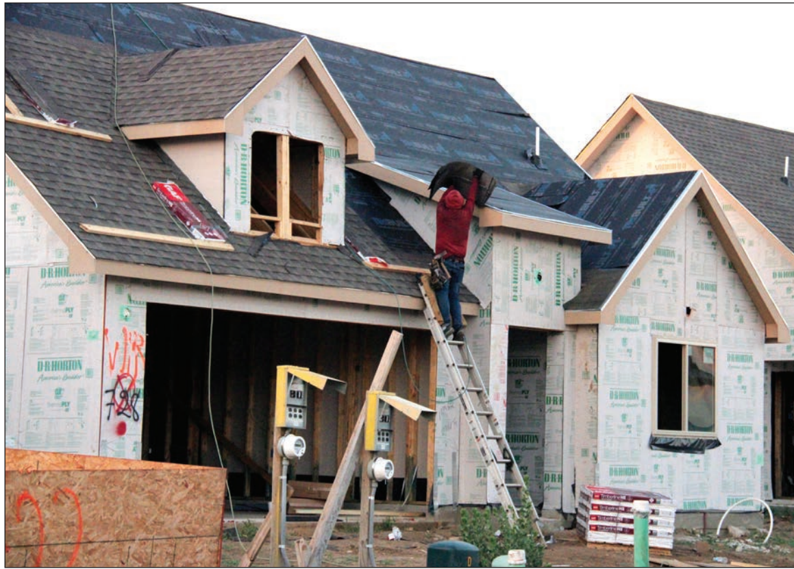
A roofer attempts to beat the heat and race the sun on a late June evening in the Windrose development north of Washington Street along U.S. 377.
