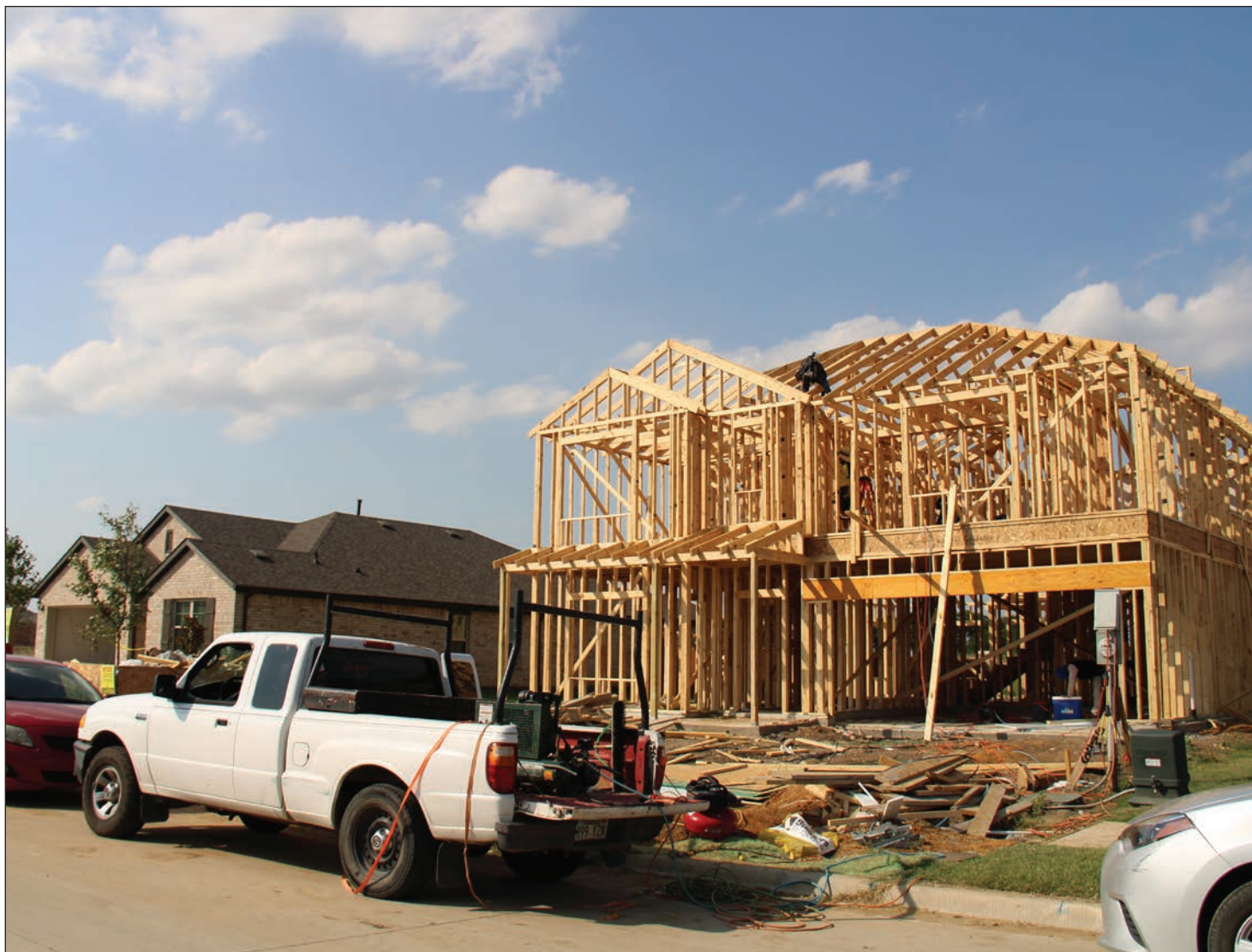
A framer works on the construction of one of the newest homes within the Mobblerly Farms development in late June. The development has rapidly been building out lots.
