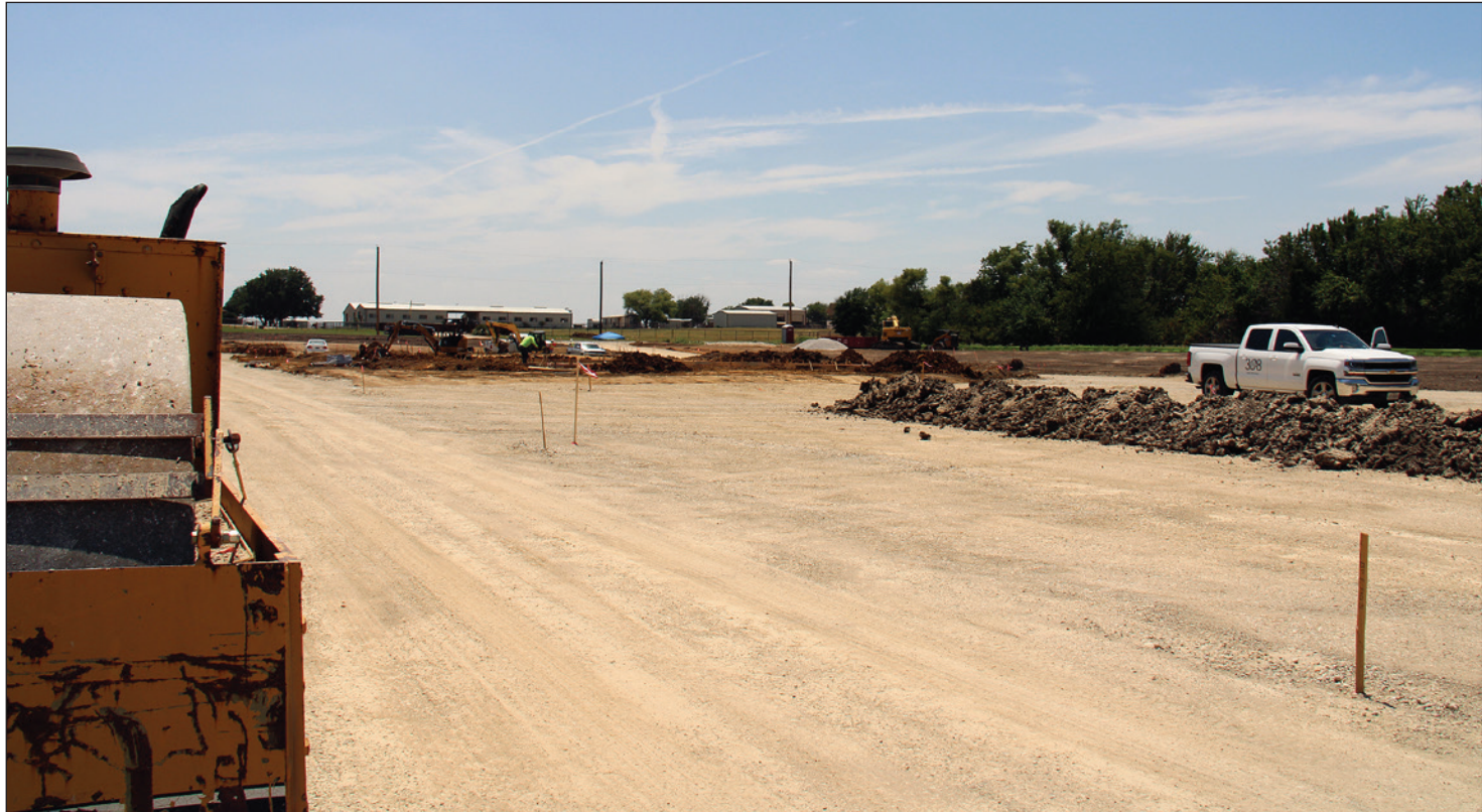
Crews work on preparing the ground for Pilot Point ISD’s new transportation center along Foutch Road in late July.
